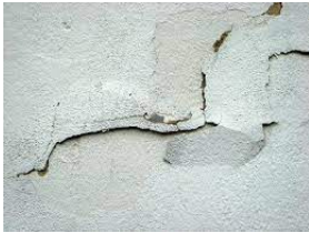
• External weak plaster
